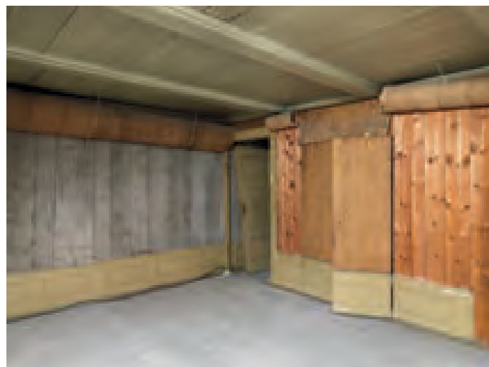
One of the north-facing rooms, room 205. The partition wall is from the beginning of the 18th century, the alcove to the right was built-in later. Photo: Roberto Fortuna.
