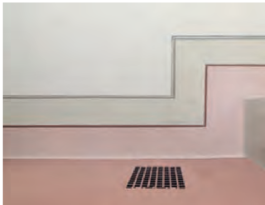
At the west end of the new first floor, the walls were painted in red with black and grey decorative lines and a trompe l'oeil skirting painted to a height of nearly half a metre. The notches were made later to help the adhesion of a plaster finish. Photo: Kurt Rodahl Hoppe. Right: Section of the ceiling decoration, 2013. Photo: Roberto Fortuna.
