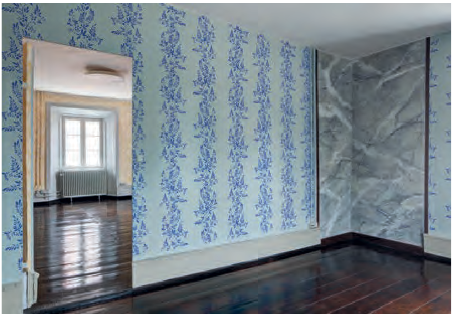
Room 209. During the restoration, all windows were thoroughly reconditioned, the openings being covered for the duration. The stove in the marbled niche had pipes to the chimney of the gable end fireplace; it no longer works, which is why no stove was put up here after the restoration. Photo: Roberto Fortuna. Bottom: Kurt Rodahl Hoppe.
