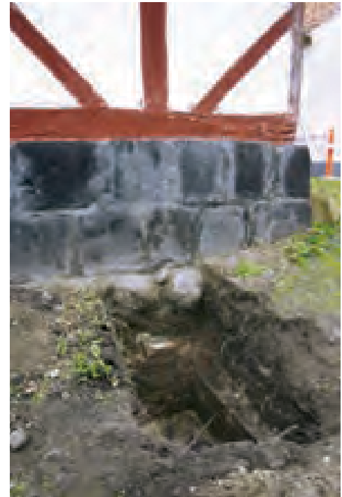
Left: The south gable end of the east wing and the corner closest to the river. Right: The continuation of the east wall of the east wing. Note the finely finished joints. City of Odense Museums.
